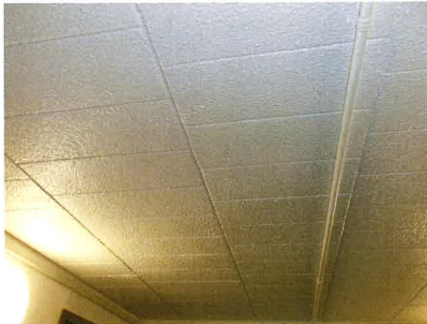
Photo 6: ACM Surfacing from Previous Survey
