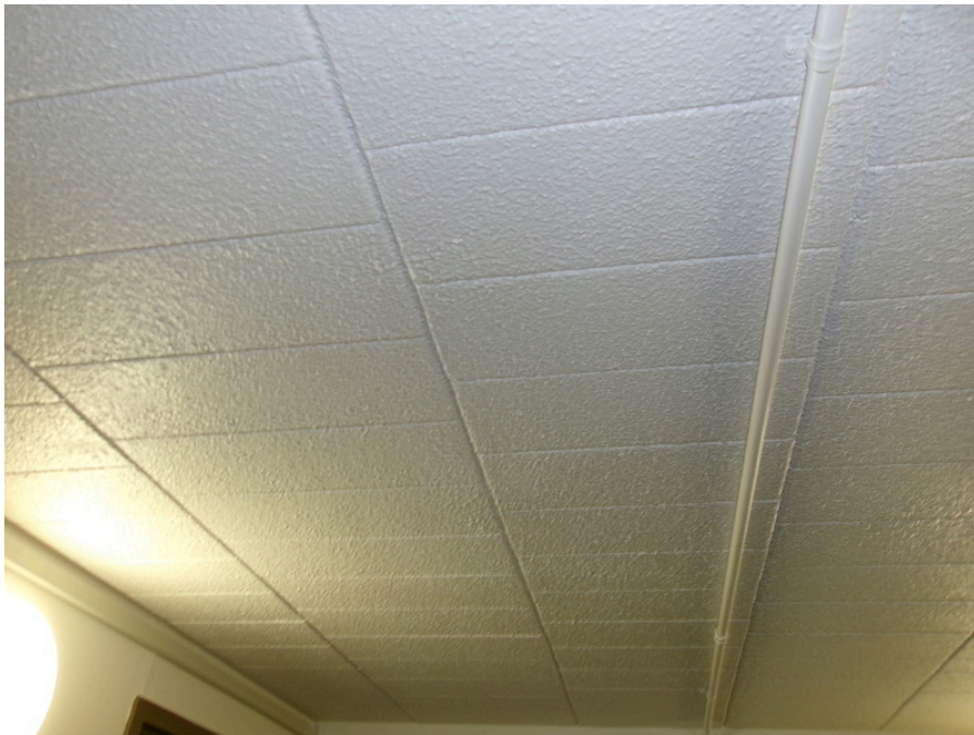
Photo 6: ACM Surfacing from Previous Survey
