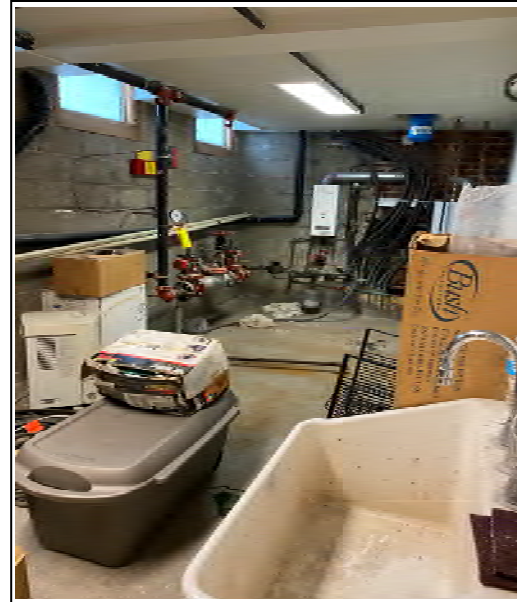
Photograph No. 18 – Basement electrical room
