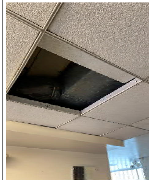
Photograph No. 34 – Ceiling tiles
