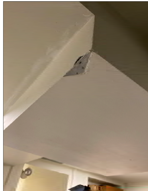
Photograph No. 12 – Ceiling plaster in basement
