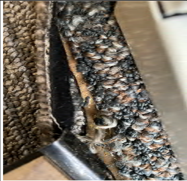
Photograph No. 5 – Wood under carpet
