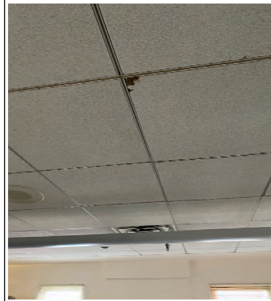
Photograph No. 30 – Ceiling tiles
