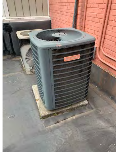
Figure 2: Split System #1 Air Condensing Unit – Annex Roof
