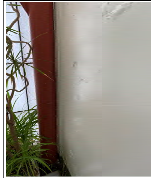
Photograph No. 26 – Damaged wall plaster and paint
