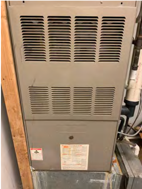
Figure 1: Split System #1 Furnace – Basement Floor
