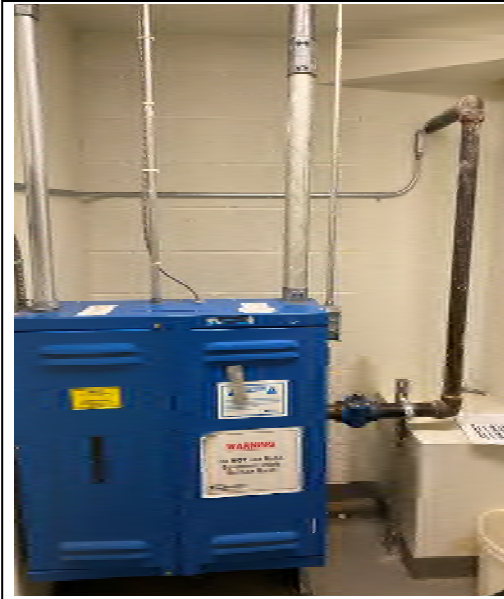
Photograph No. 13 – Pipe insulations
