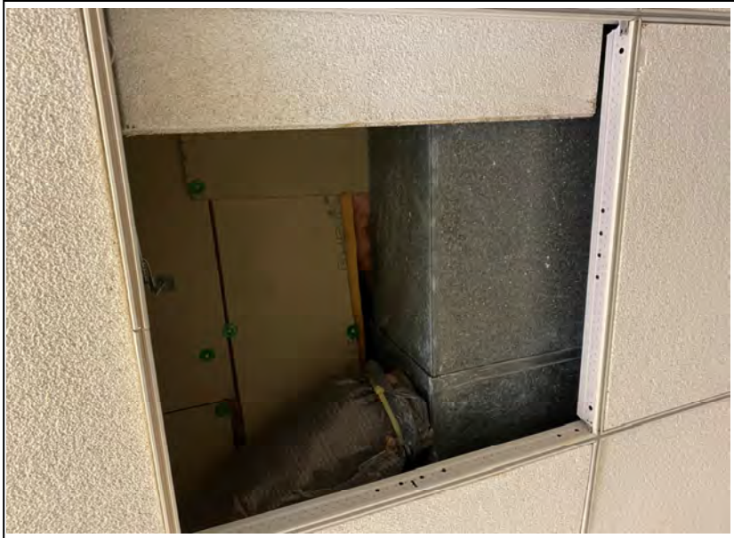
Photograph No. 1 – 3rd floor ceiling tiles
