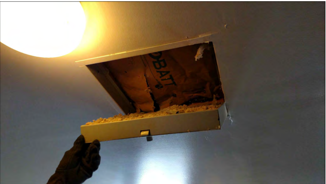
1310 FERRIS LOCATION SMALL ACCESS PANEL INACCESSIBLE 12
