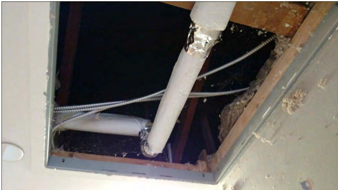
1310 FERRIS LOCATION ACCESS HATCH AND SPRINKLER PIPING 11
